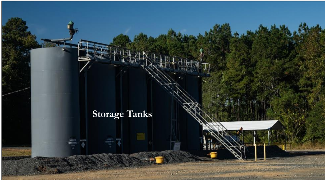
Typical wellsite in Terryville
