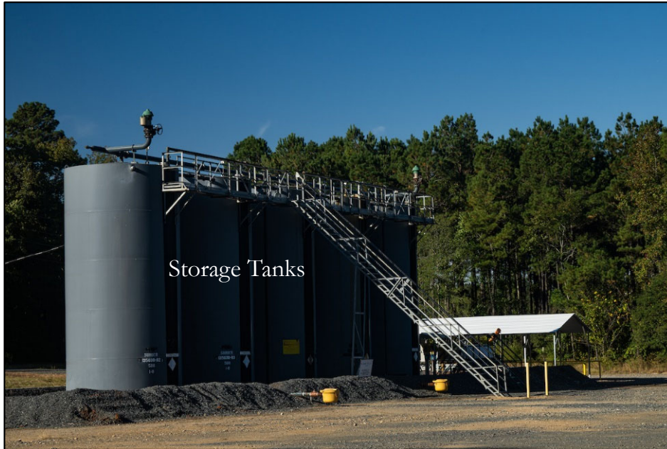
Typical wellsite in Terryville
